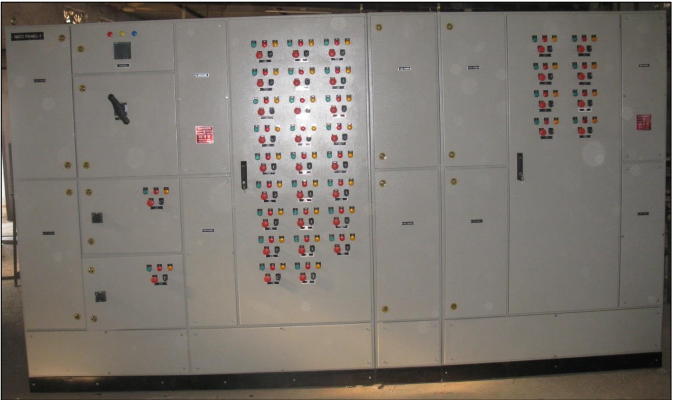
Fig: Front View panel-With doors closed
